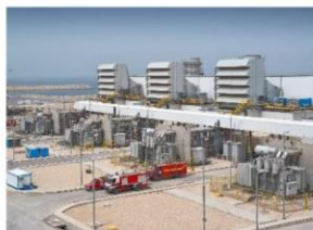
Combined power plant 1130 MW
