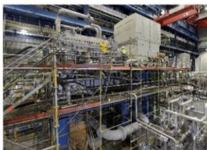
String test of pre-cooling compressor
