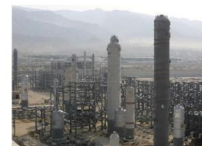
Equipment & structures, treating units
